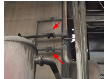
These valves must be locked out before Welding in new 3" isolation for Downcomer spill
